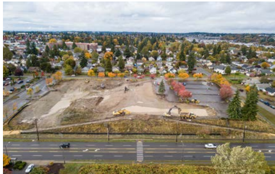
South Sound 911's future public safety communications center (PSCC) will be built at 3580 Pacific Ave., shown above on Oct. 20, 2017.
